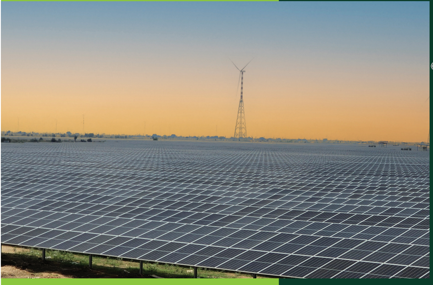
ReNew 400 MW Site Jaisalmer, Rajasthan
