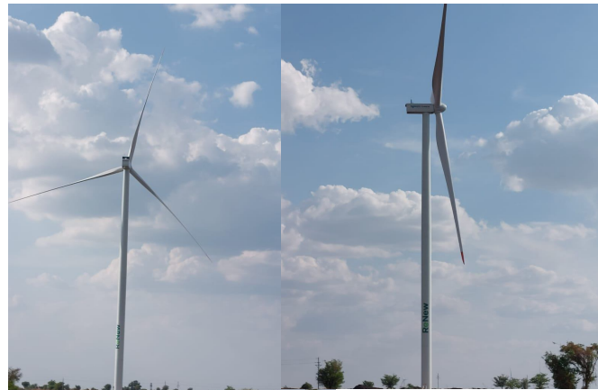
Round the Clock (RTC) Power Project
